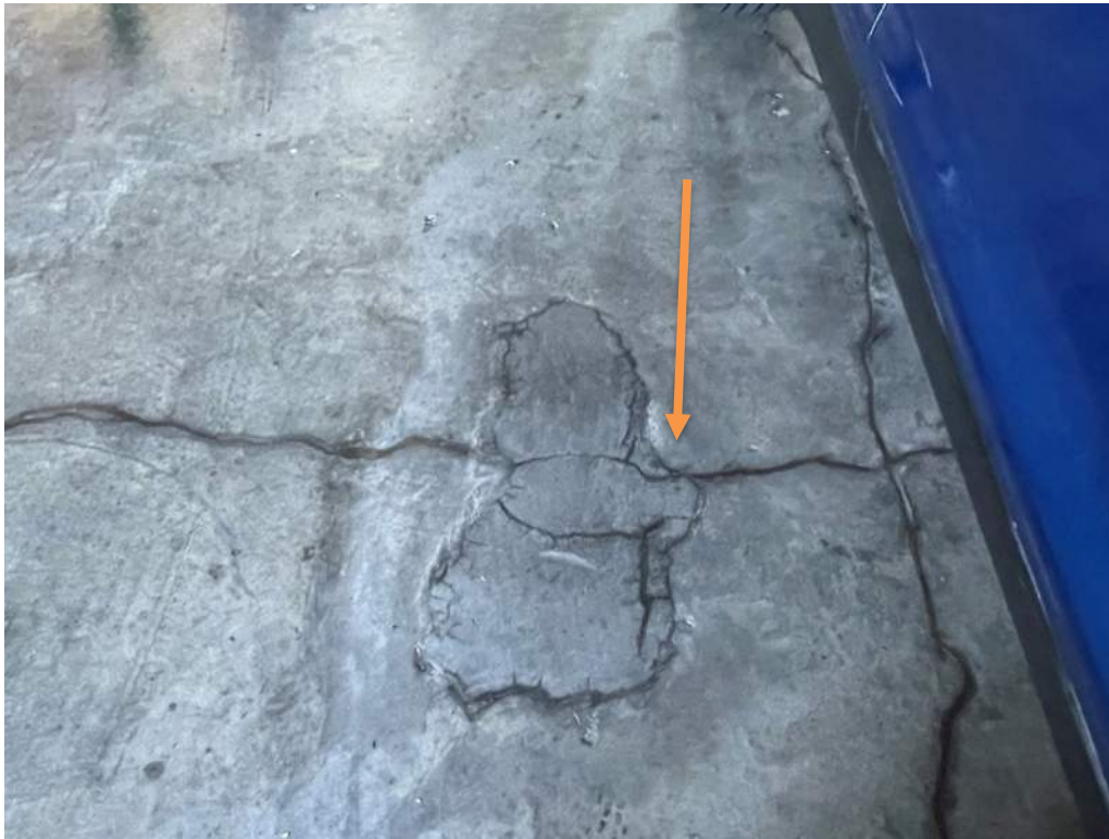
Figure 49 – Parking garage slab cracks and typical previous repair
