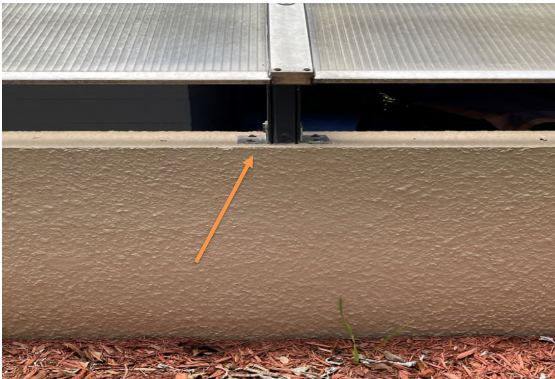
Figure 27 – Evidence of water intrusion at unsealed corroded fasteners on exterior wall of parking garage
