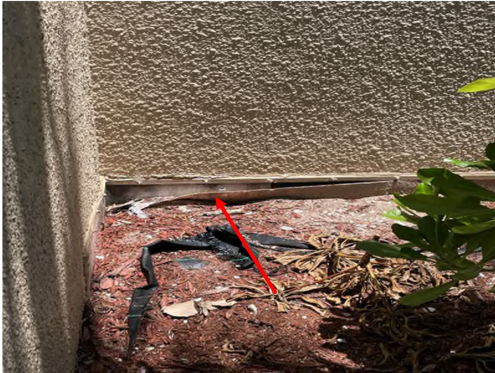
Figure 28 – Possible moisture issue
