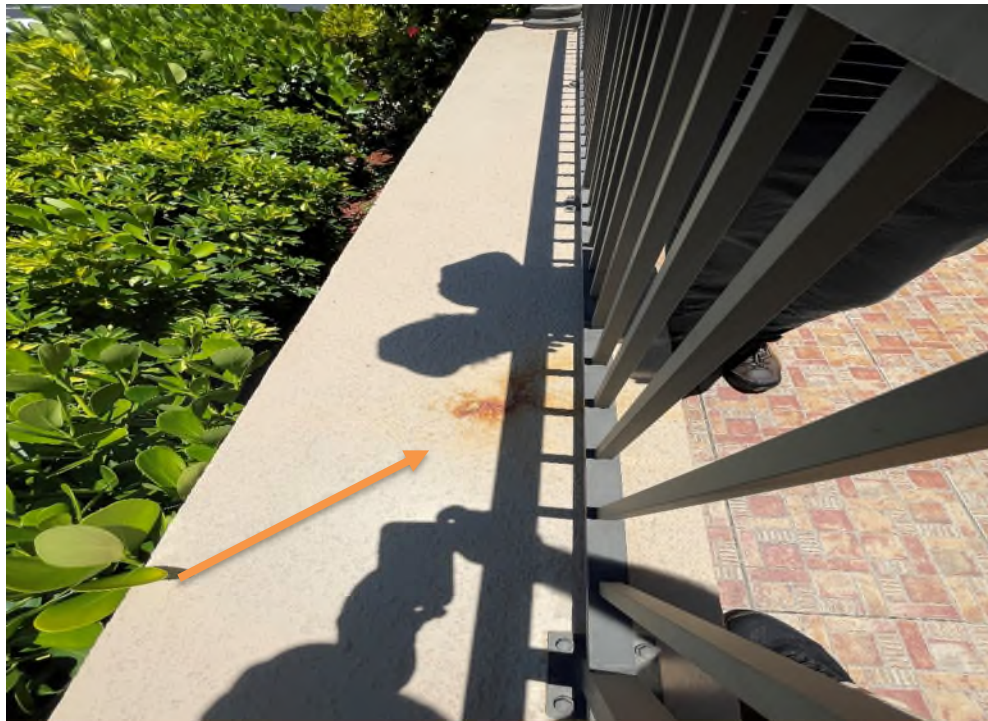
Figure 35 – Possible corrosion on railing system – staining of wall under front entrance railing system.
