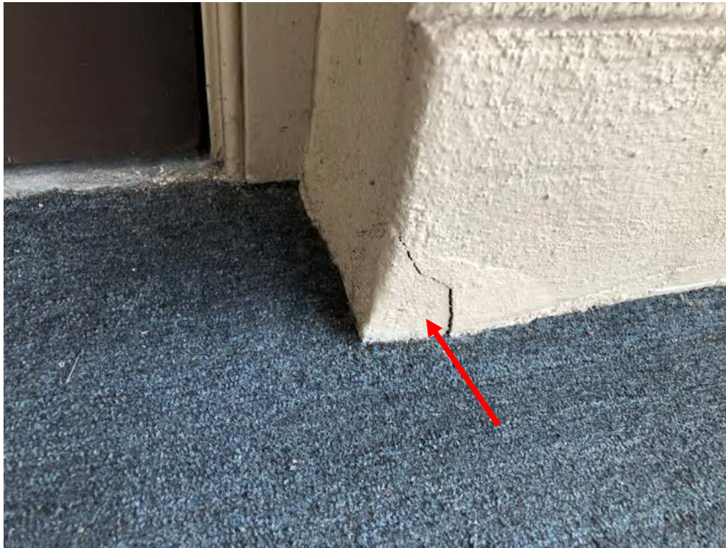
Figure 10 – Stucco crack on balcony wall Unit 533
