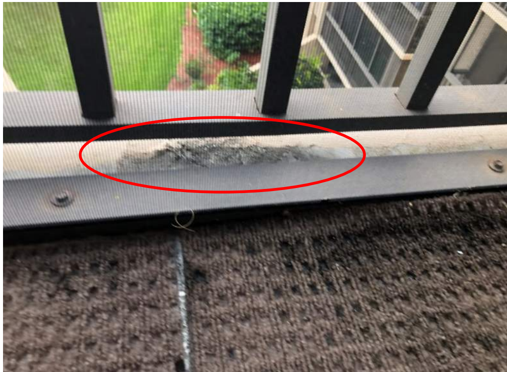
Figure 42 – Typical coating delamination at balcony slab edge under railings - Unit 512
