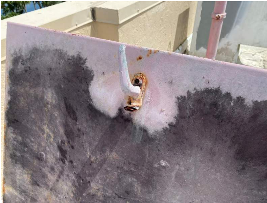
Figure 25 – Corroded Roof access
