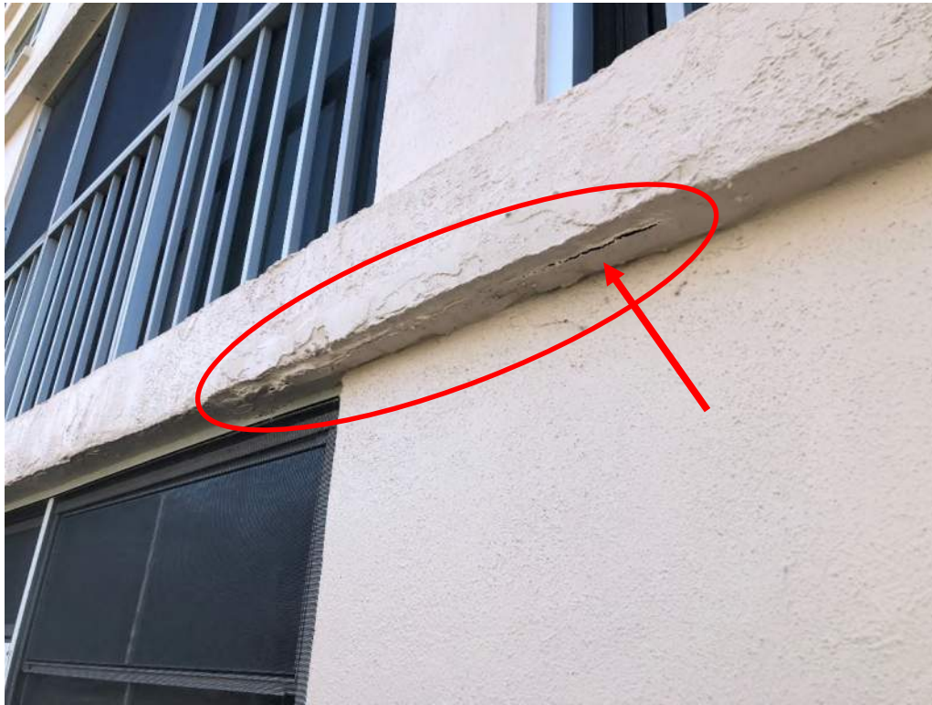
Figure 5 – Spalling on balcony slab edge
