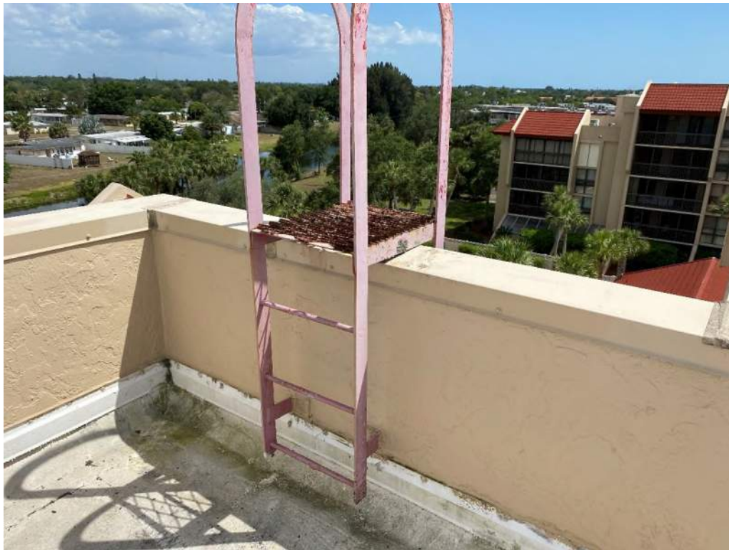
Figure 24 – Existing condition of the steel ladder on the roof
