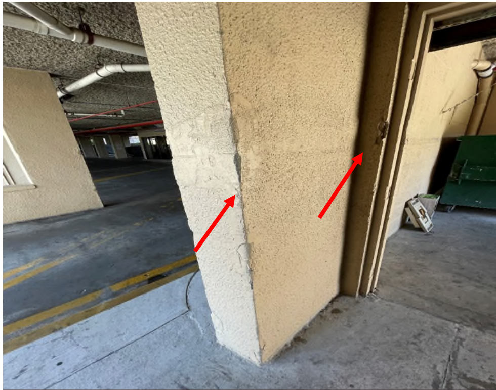
Figure 13 – Existing areas needing repair along the CMU wall located near trash room
