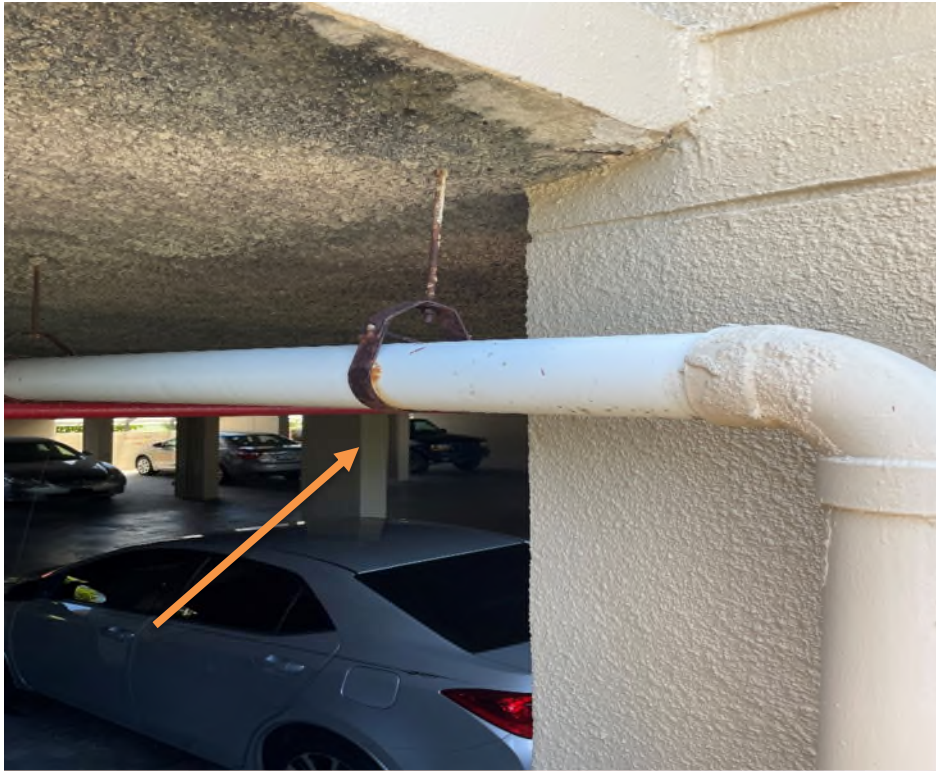
Figure 51 – Typical rusted pipe hangers, anchor bolts, and fasteners throughout parking garage.
