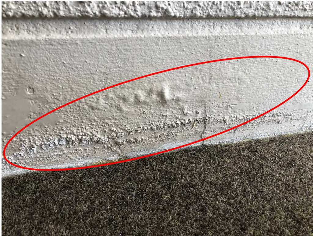
Figure 44 – Deterioration observed along balcony wall - Unit 5
