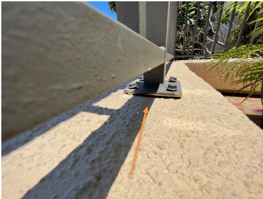
Figure 37 – Fasteners not fully seated on front entrance railings
