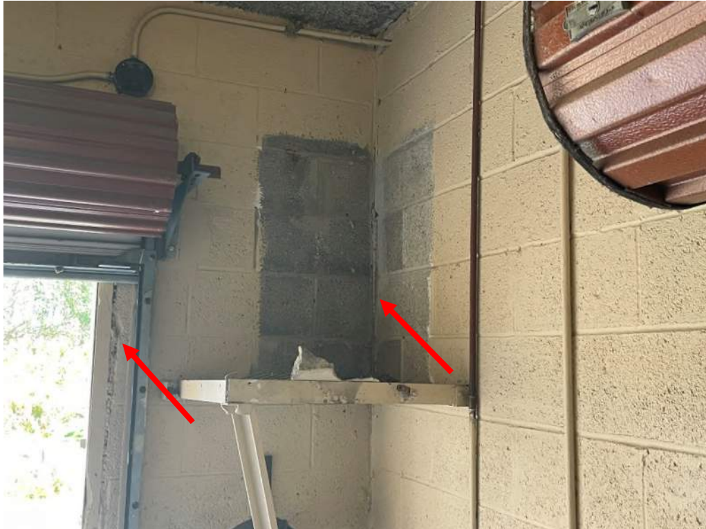
Figure 14 – Cracks and voids identified on the interior walls of the trash room
