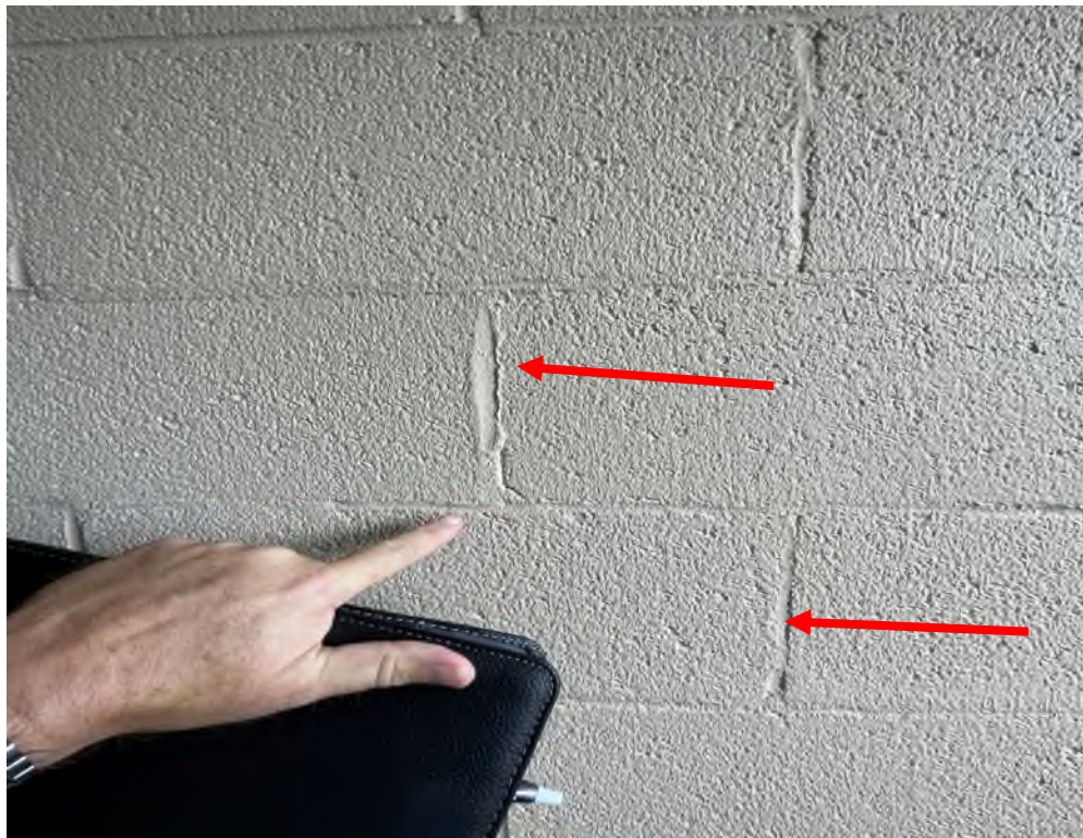
Figure 12 – Identified Stair stepping cracks located in the parking garage. Near Parking Spot 148.
