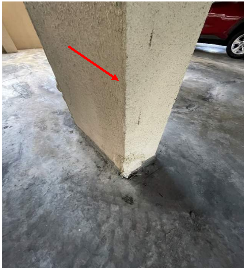
Figure 9 - Identified spalling in parking garage
