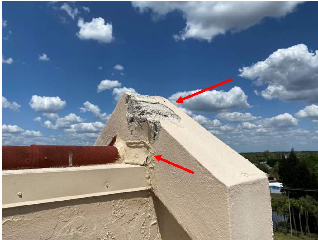
Figure 22 – Damage susceptible to water intrusion
