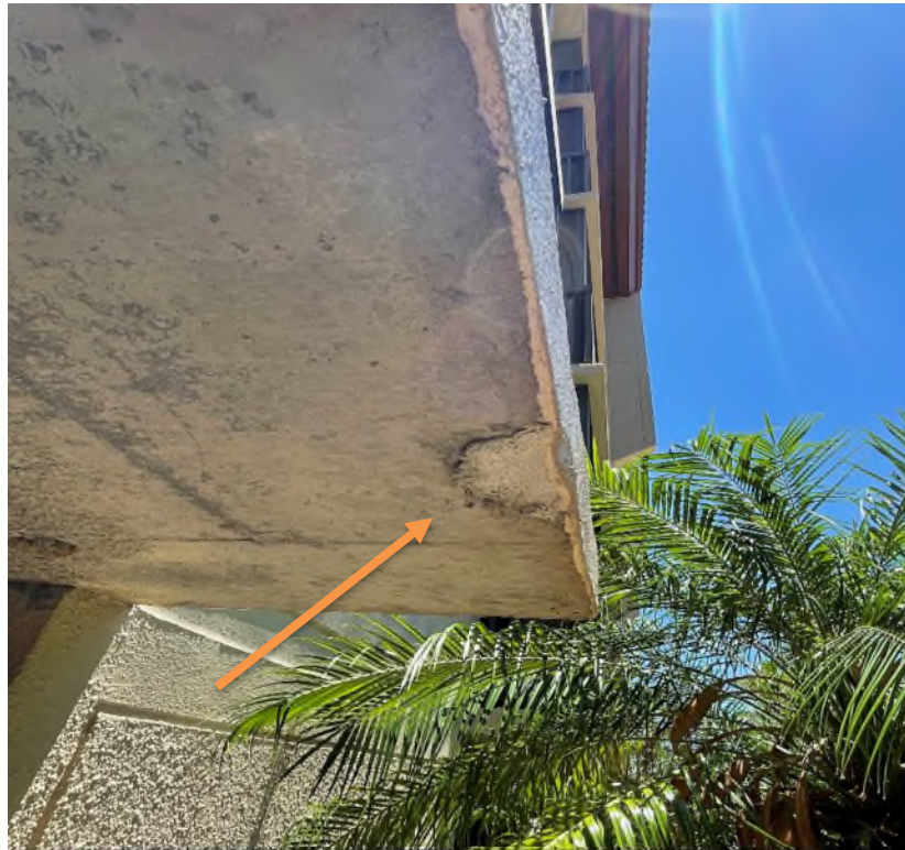
Figure 1 – Spalling at the parking garage ceiling East side near clubhouse
