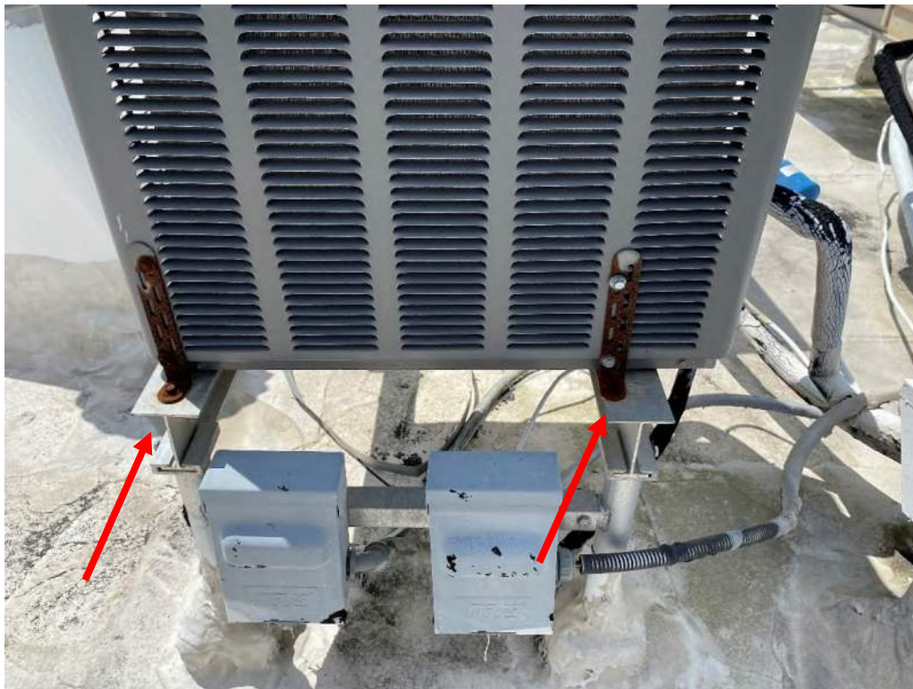
Figure 20 – Typical oxidated A/C tiedowns
