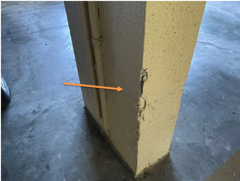
Figure 50 – Typical column damage throughout parking garage.
