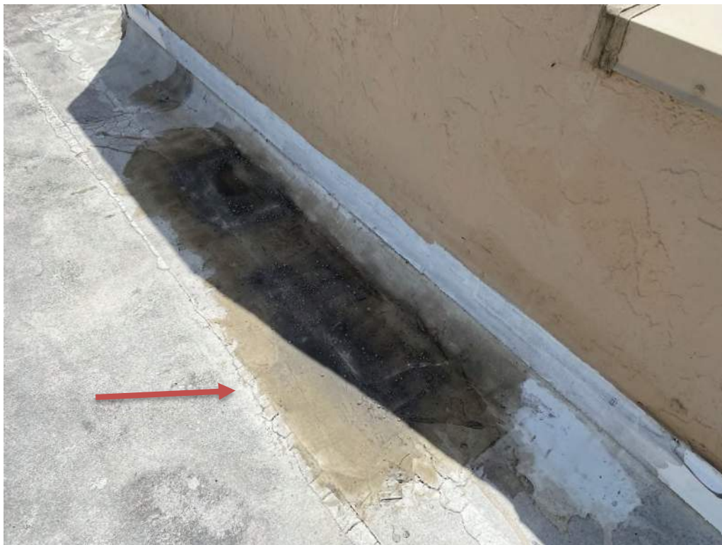
Figure 23 – Evidence of water ponding
