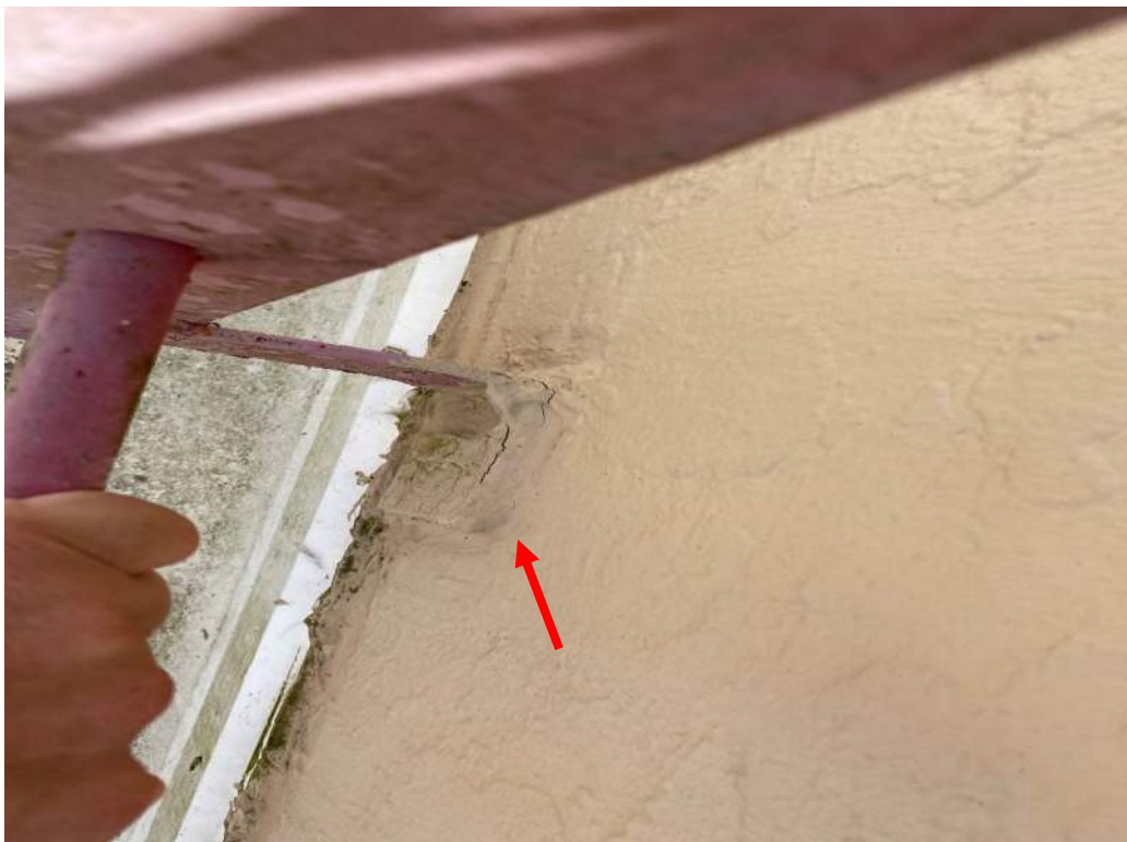
Figure 26 – Mount failing at wall to ladder attachment area
