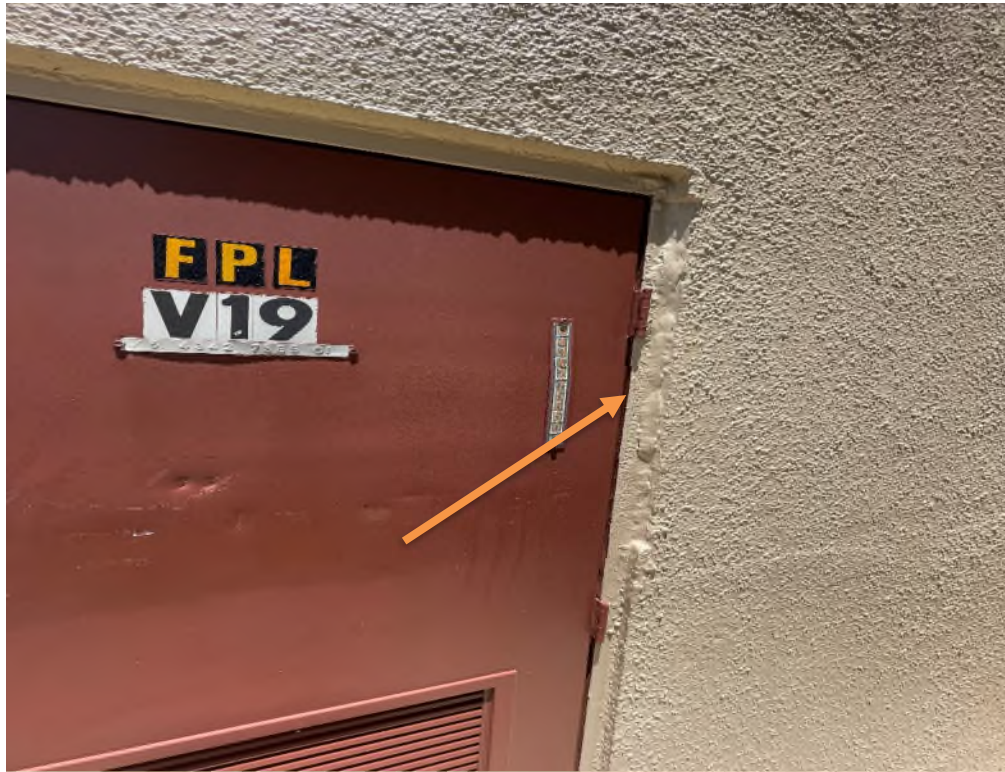
Figure 31 – Failed sealant along exterior door
