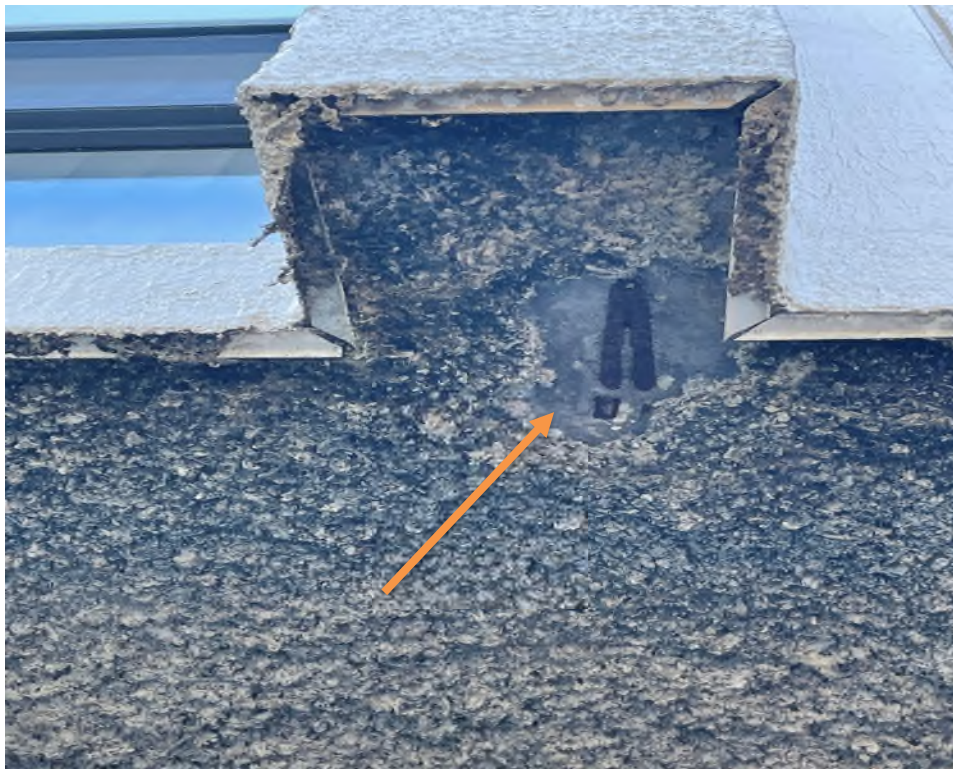
Figure 46 – Stucco delamination and exposed rebar found at the North Entrance
