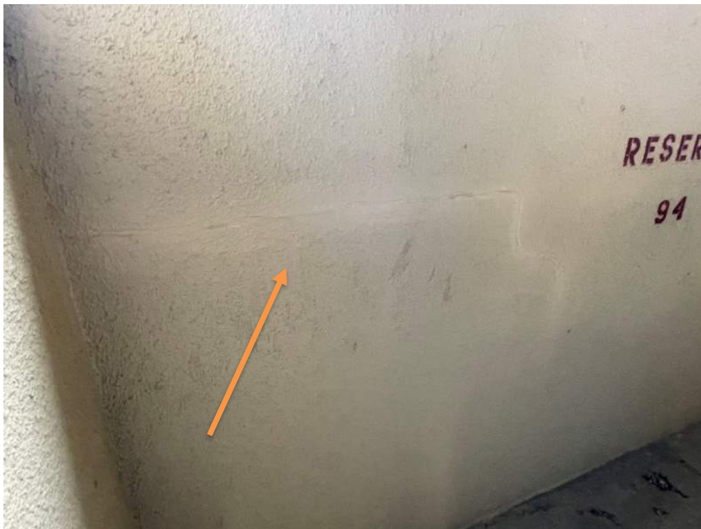
Figure 48 – Typical stair step cracking on parking garage wall
