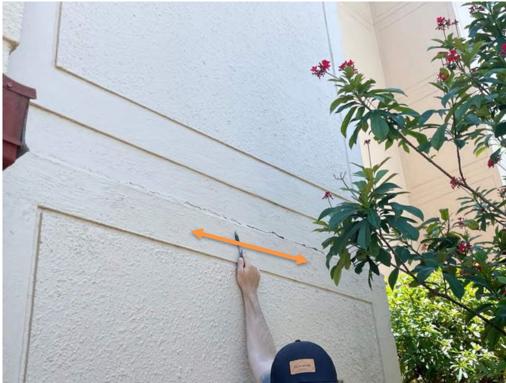
Figure 3 – crack repair needed near front entrance of Promenades East
