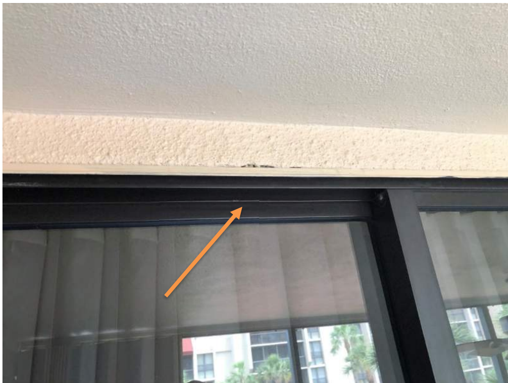
Figure 32 – Failed sealant or lack of sealant around sliding glass doors
