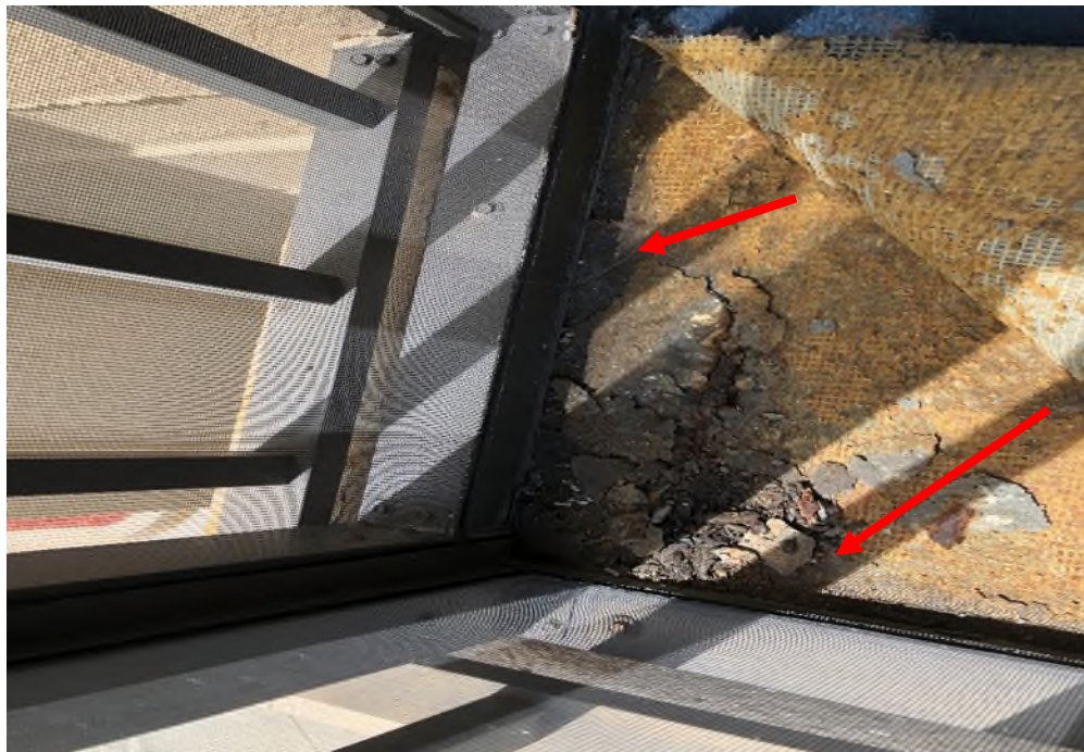
Figure 36 – Deterioration – Railing to Balcony Slab – Unit 309
