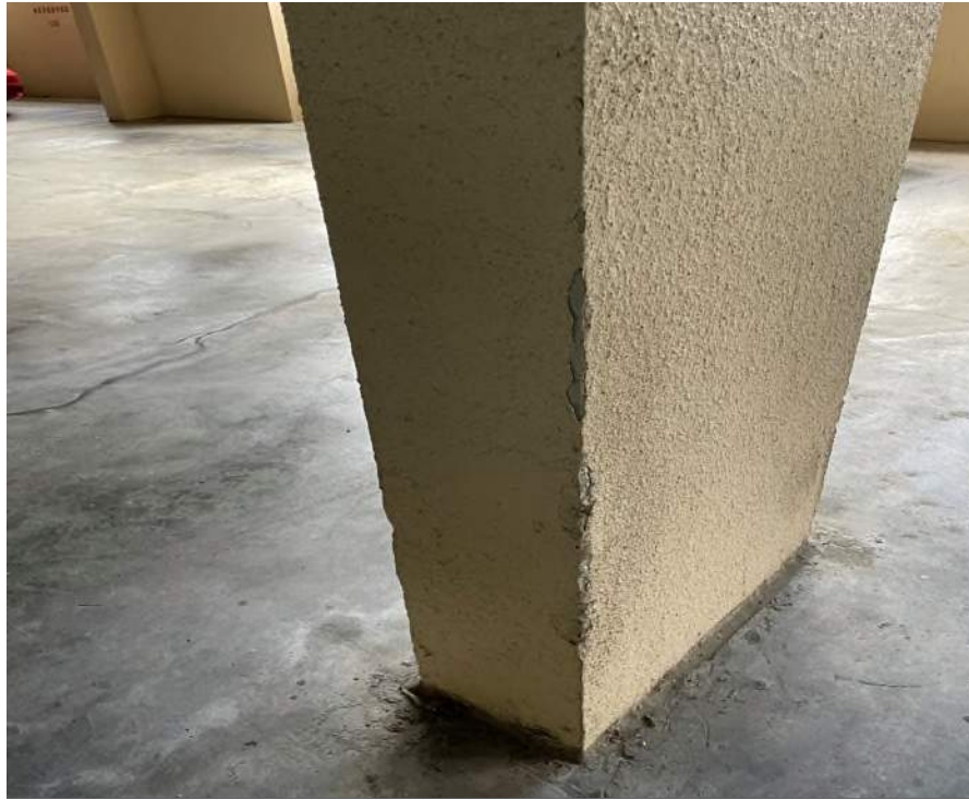
Figure 7 – Stucco delamination identified at exterior column
