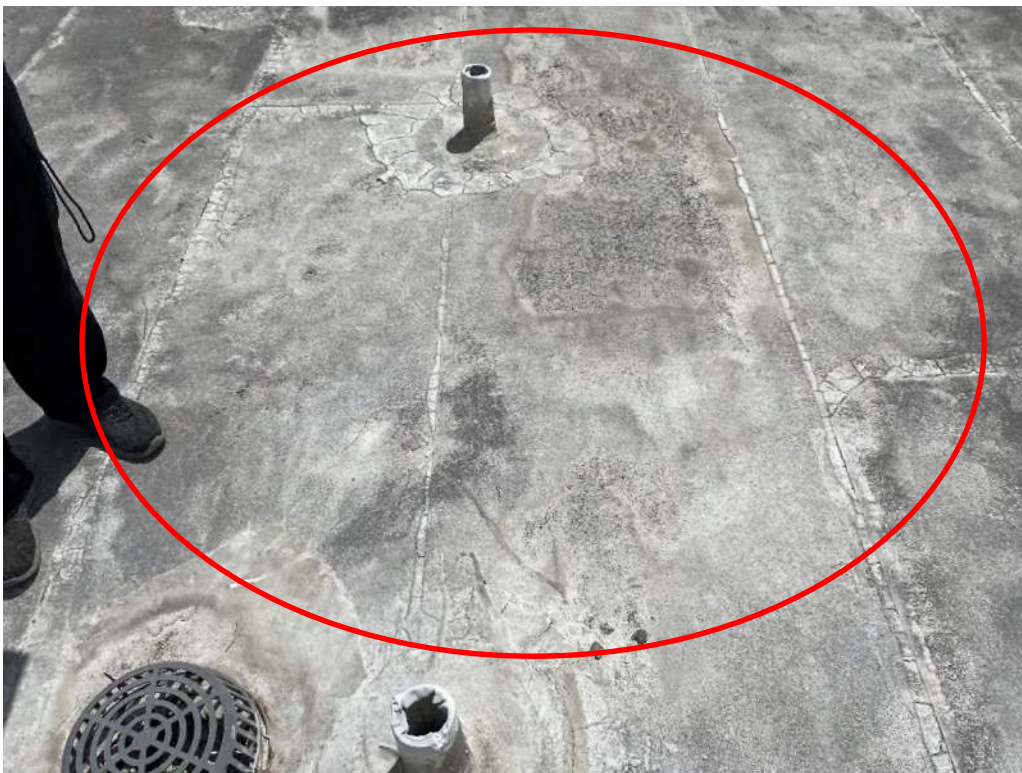
Figure 19 – Roof at end of life – cracks in membrane
