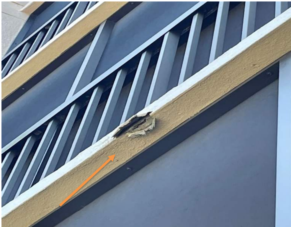
Figure 2 – Spalling on balcony slab edge
